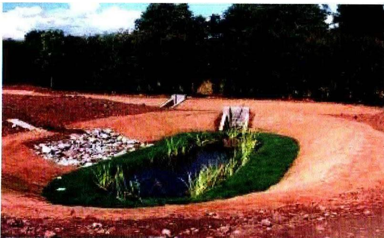
Photograph of the Makria reservoir, which is an important freshwater habitat today, west of Limassol New Port and part of the Milton Street storm water drainage project.
